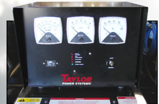
Analog Generator Control Panel
