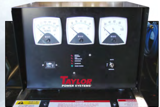
Analog Generator Control Panel
