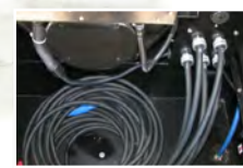
Storage Area for Output Cables
