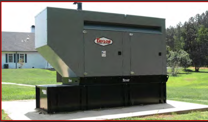
■ DIESEL & GAS STANDBY GENERATORS
